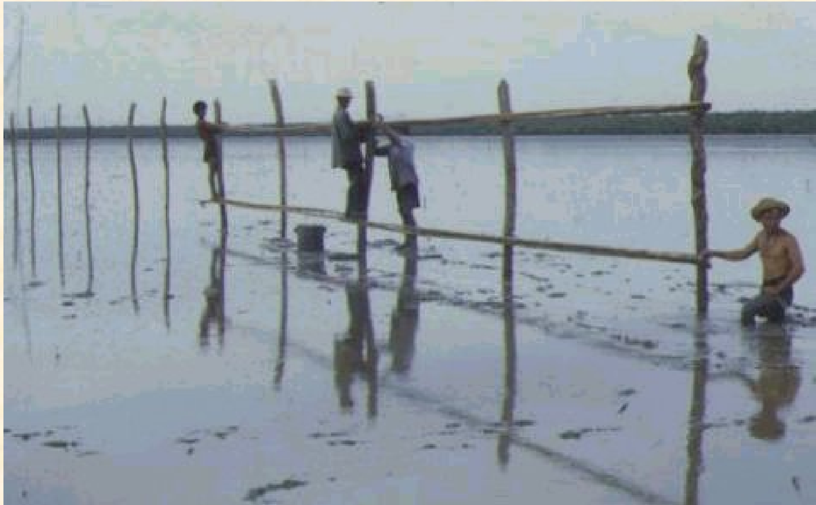
Building a 9-km fence round a replanted mangrove, Samut Songkram, Thailand ( Photo: WWF )
