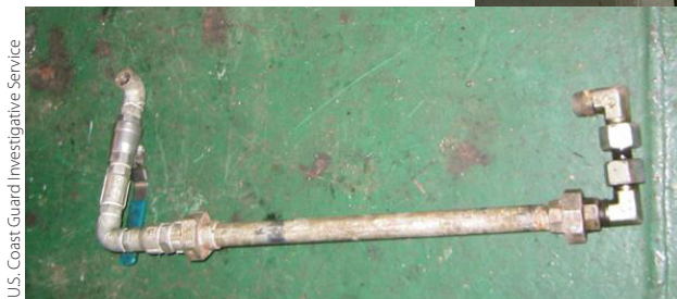
13. Fabricated piping with oil residue found in storeroom.
