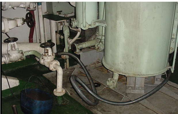
15. Marine Sanitation Device showing overboard sewage discharge piping.
