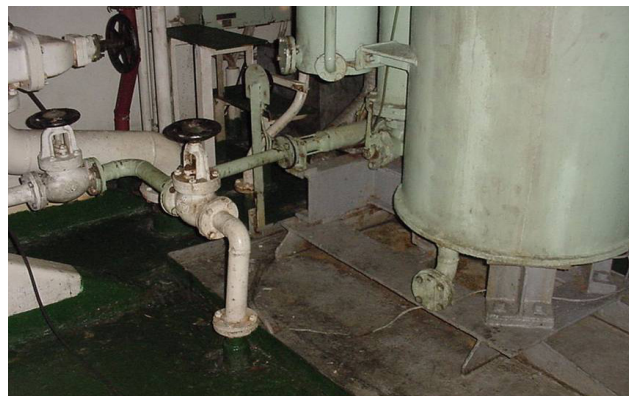
16. Bypass hose connecting bilge piping to Marine Sanitation Device discharge piping.
