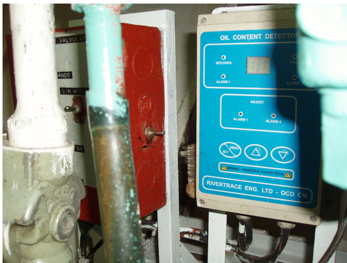
21. Bypass switch installed to silence the Oil Content Monitor alarm and allow the Oily Water Separator to continue to operate even when oil content is more than 15 ppm.
