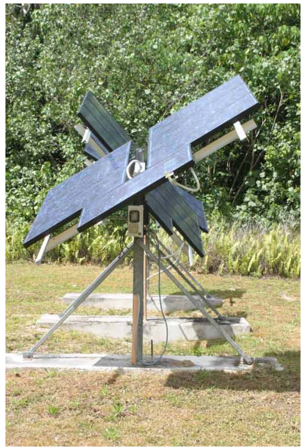
Figure 4-2 - Sun tracking PV panels for solar pump (inoperative)
