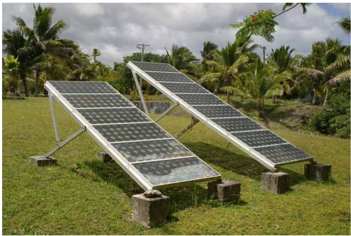
Figure 4-1 - Panels for Namukulu Community Hall (note corrosion and delamination of the lower panels)
