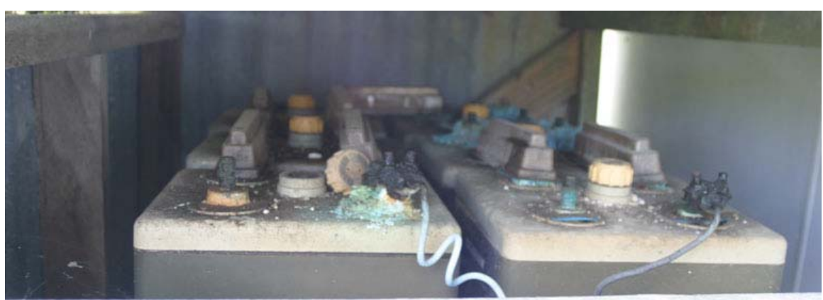
Figure 7-1 - Failed batteries at Namukulu village still good for recycling after 10 years of storage
