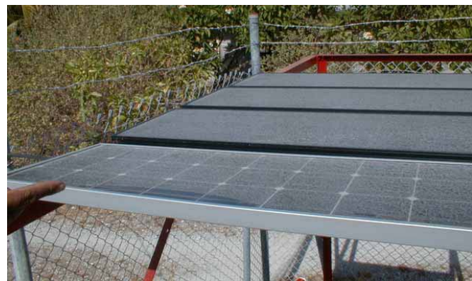
Figure 4-1 - Marakei telecom installation (note the surface dirt)
