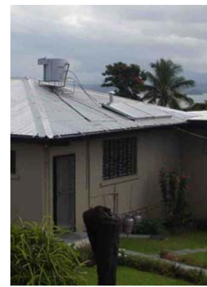
Figure 5-12 – Beasley Solar Water Heater, Suva
