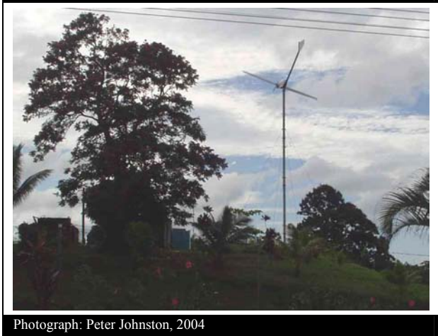
Figure 5-21 – Small Wind Electric System, SOPAC, Suva
