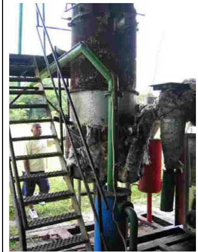
Figure 4-3 – Derelict Gasifier, Onesua
