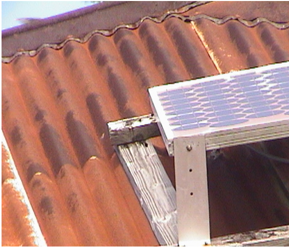
Fig 3: A Mango installation (1991) Roof Mounted; other PV components inside
