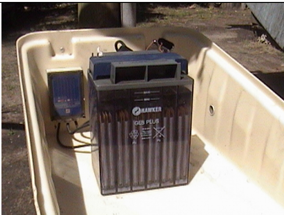
Fig 5: A Kotu installation (2002). Pole mounted panels. Controller and battery in a box attached to the pole.
