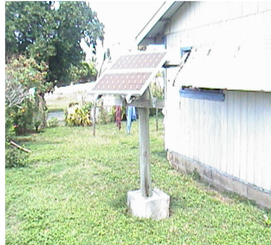
Fig 4: A Mo'unga'one installation (1994). Pole Mounted; other PV components Inside
