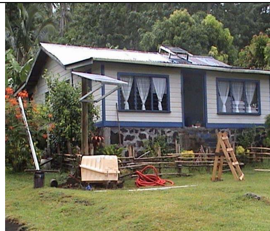
Fig 6: A Niufo'ou installation (2006) Pole mounted panels. Controller and battery in a box attached to the pole.
