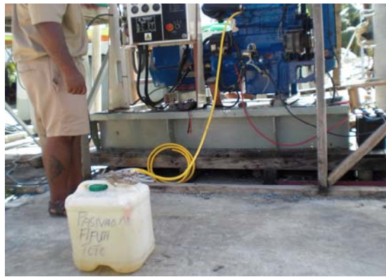
Fig 21: Testing of bio-diesel with the generator
