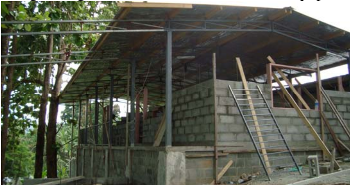
Side view of the building from where the biodiesel generator will be set-up
