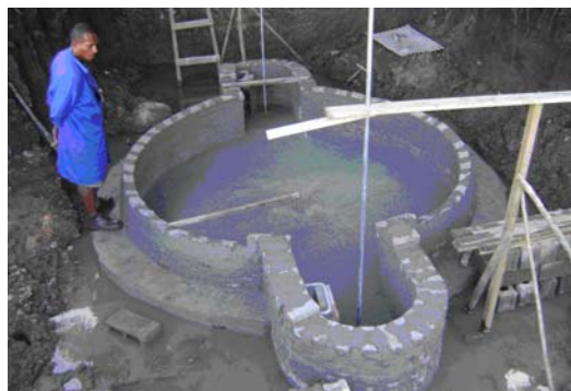
8m 3 Digester- Namatakula
