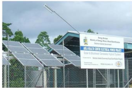
A Hybrid System installed at AOLA Rural Health Centre (North Guadalcanal)
