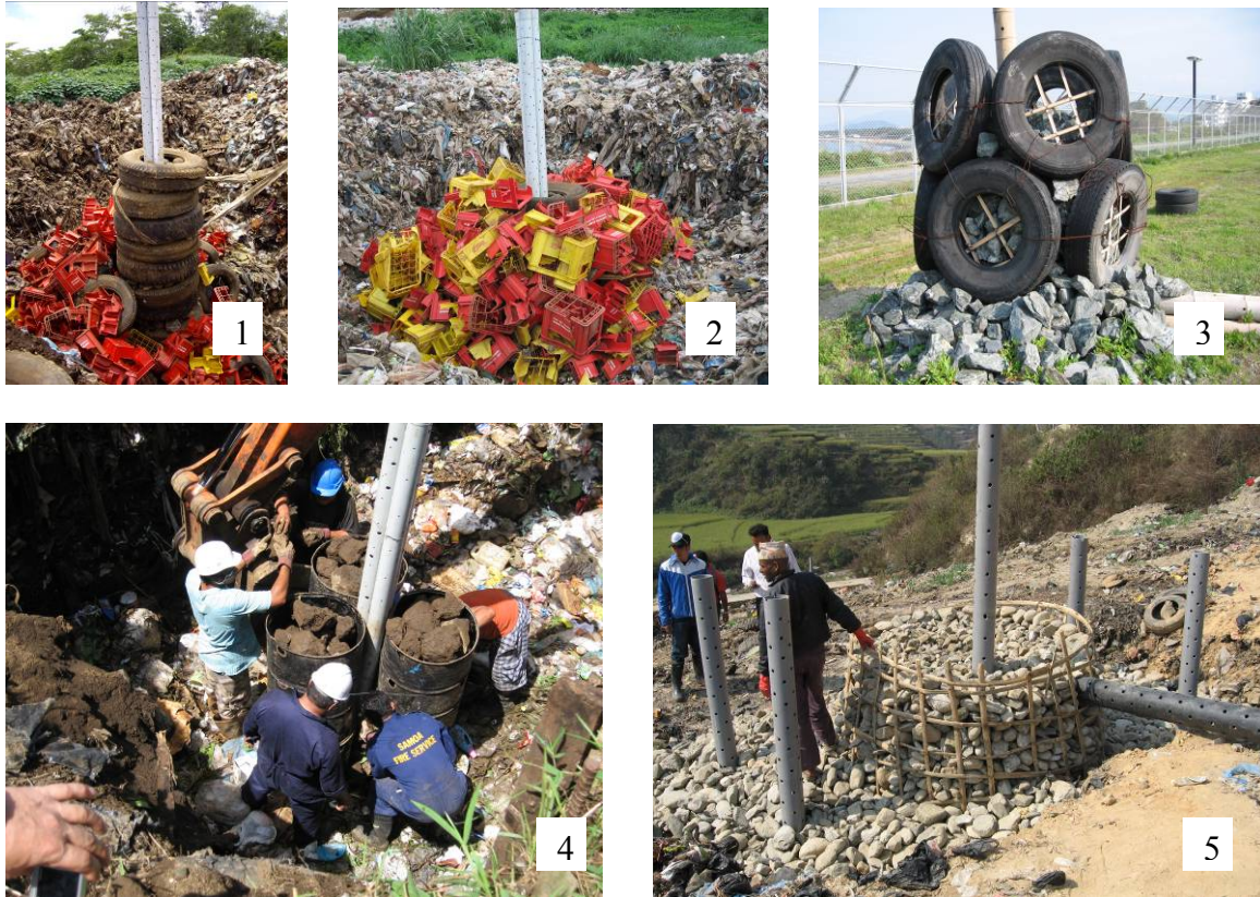
Photo- 29: Different Types of Vertical Gas Venting Facility to Enlarge the Aerobic Zone around the Pipe
