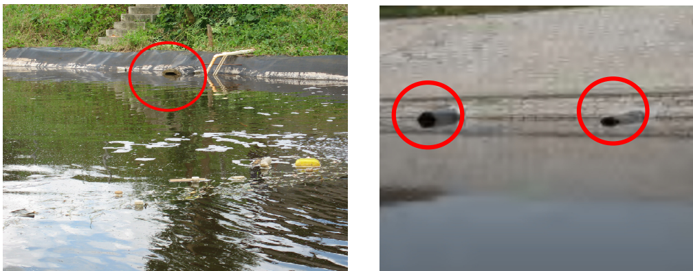
Photo- 39: Submerged leachate pipe outlet (example of bad practice)
