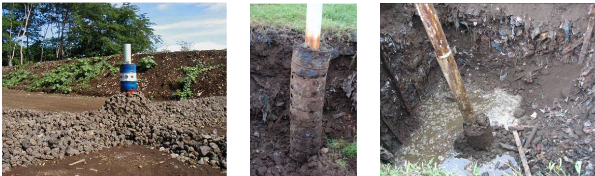
Photo- 26: Vertical Gas Venting Pipe installed on Pipe Connection Pit
