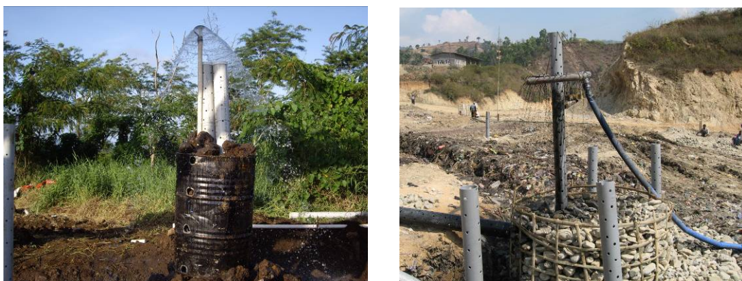
Photo- 31: Various types of Treatment System (Trickling Filter) for Re-circulation
