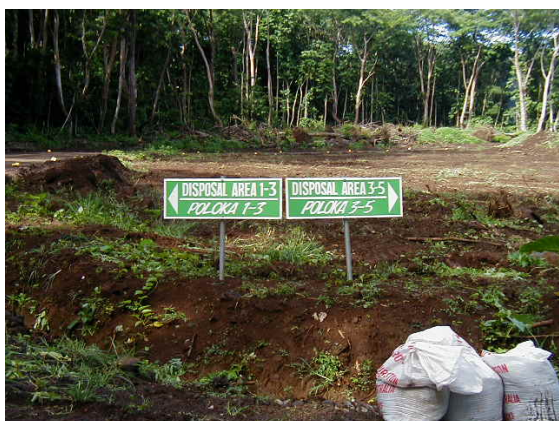
Photo- 34: Sign Boards on Access Road
