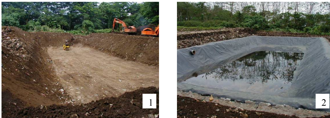
Photo- 23: Leachate Retention Pond
