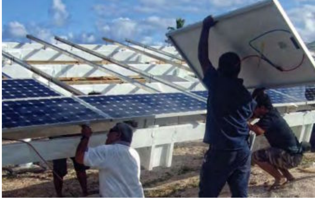
EU-funded photovoltaic systems in Niue PHOTO – PIGGAREP
