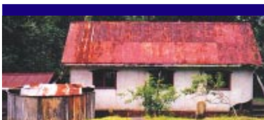
Corrosion of roof catchment from salt spray and volcano-induced acidic rain
