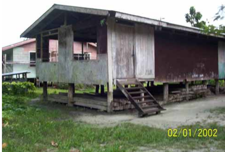
Plate 4: Dilapidated school building at Mbili Passage
