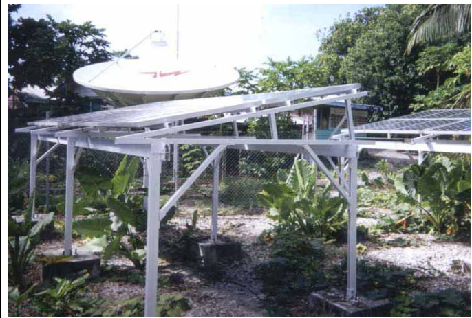
Figure 4-2 – USP Solar Installation Atafu
