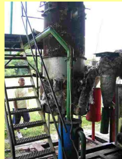
Figure 4-3 – Derelict Gasifier, Onesua
