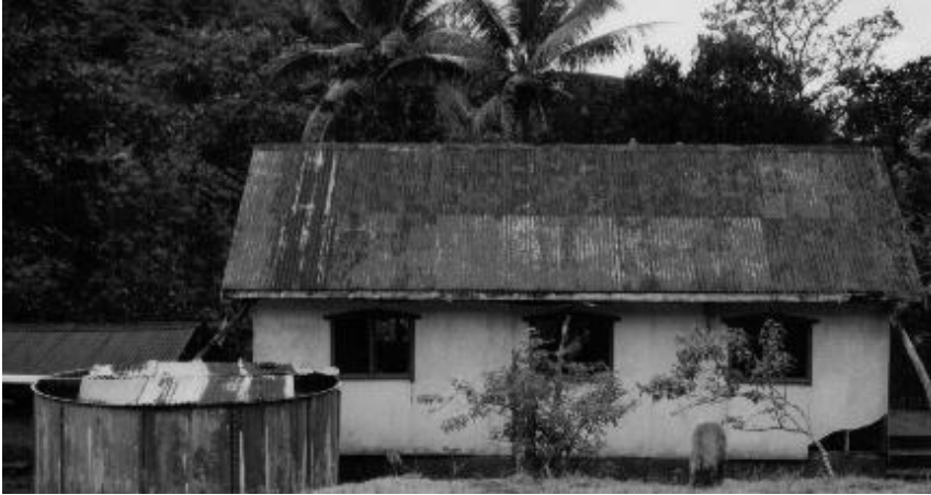
Fig: 14. Corrosion of roof catchment from salt spray and volcano induced acidic rain
