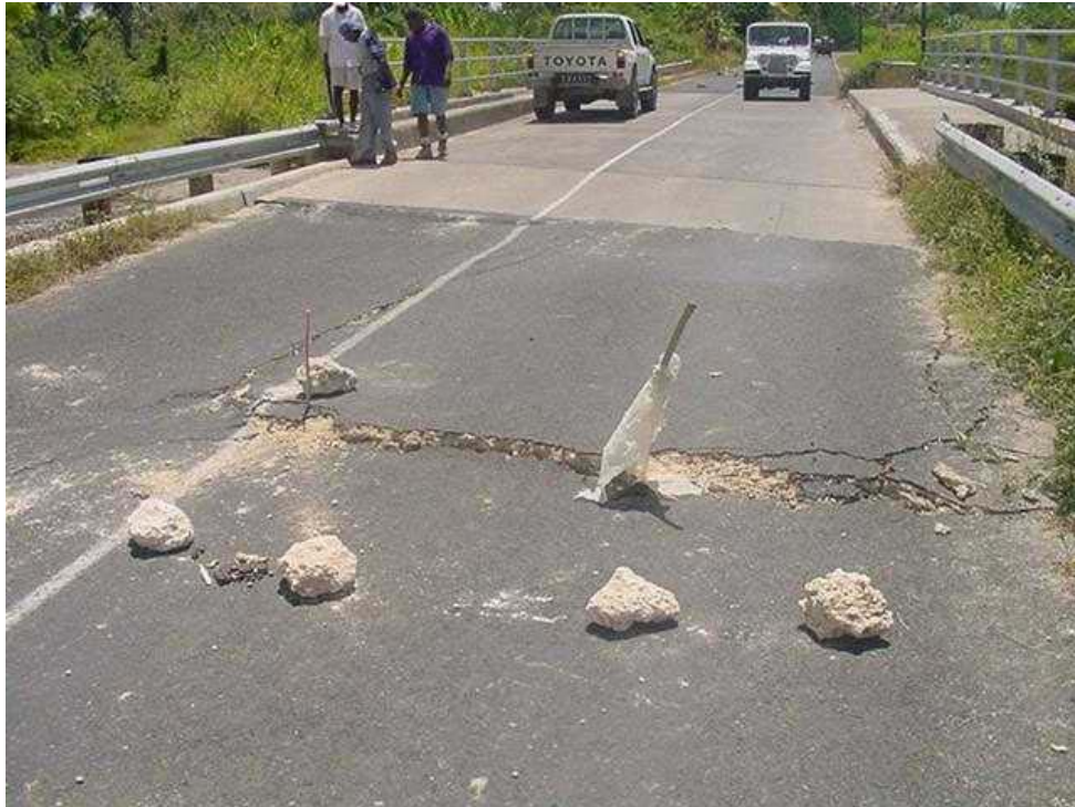
Road infrastructure damage during earthquake in the year 2002.
