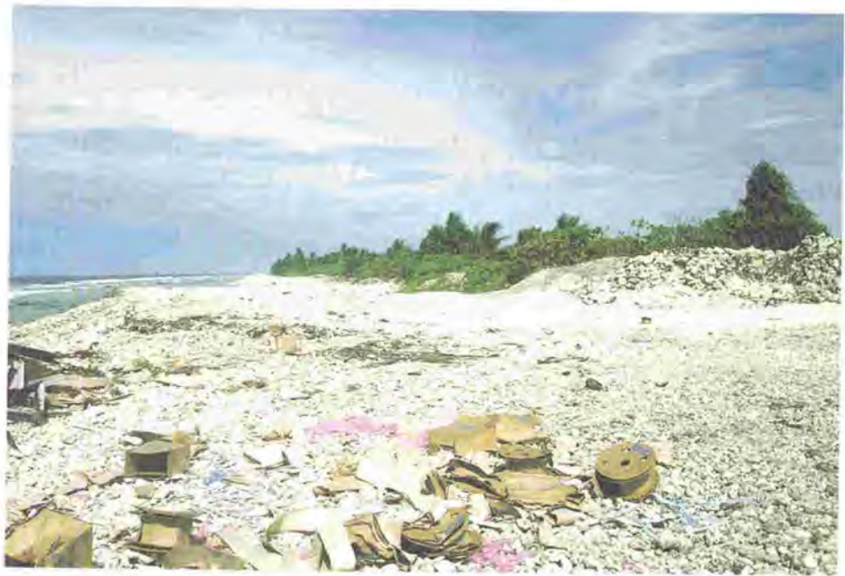
Crushed rock for construction is excavated from the ocean foreshore, thus reducing the protection offered by the natural "sea wall" built by Cyclone Bebe. (photo: Alefaio Semese)
