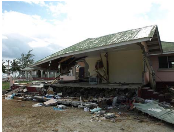
Figure 44: Damage in Poutasi
