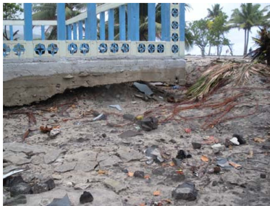
Figure 45: Large sections of the foundation are undermined
