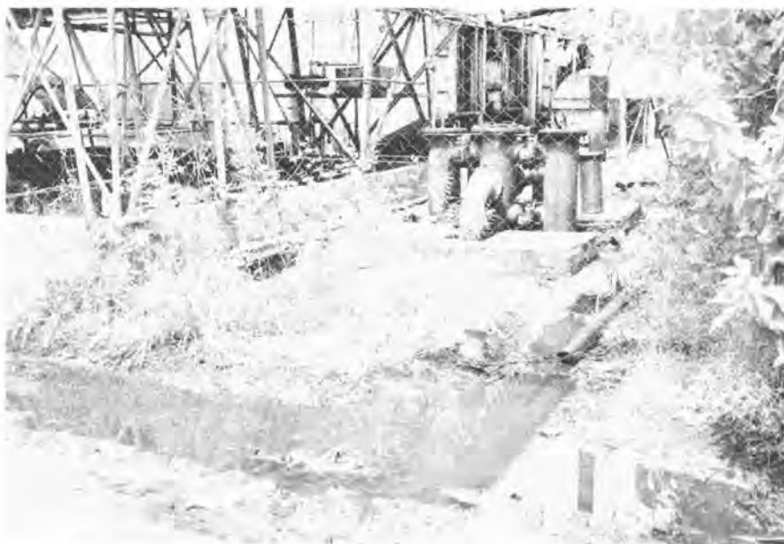
Oil contamination at the Betio powerhouse. Continual small-scale discharge could result in groundwater contamination. (photo: Craig Wilson)
