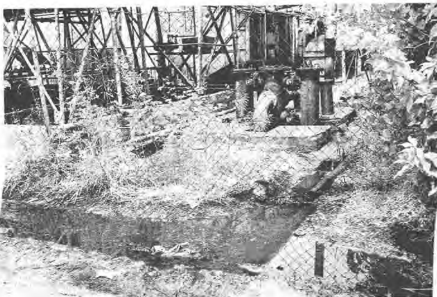
Oil contamination at the Betio powerhouse. Continual small-scale discharge can result in groundwater contamination. (photo: Craig Wilson)
