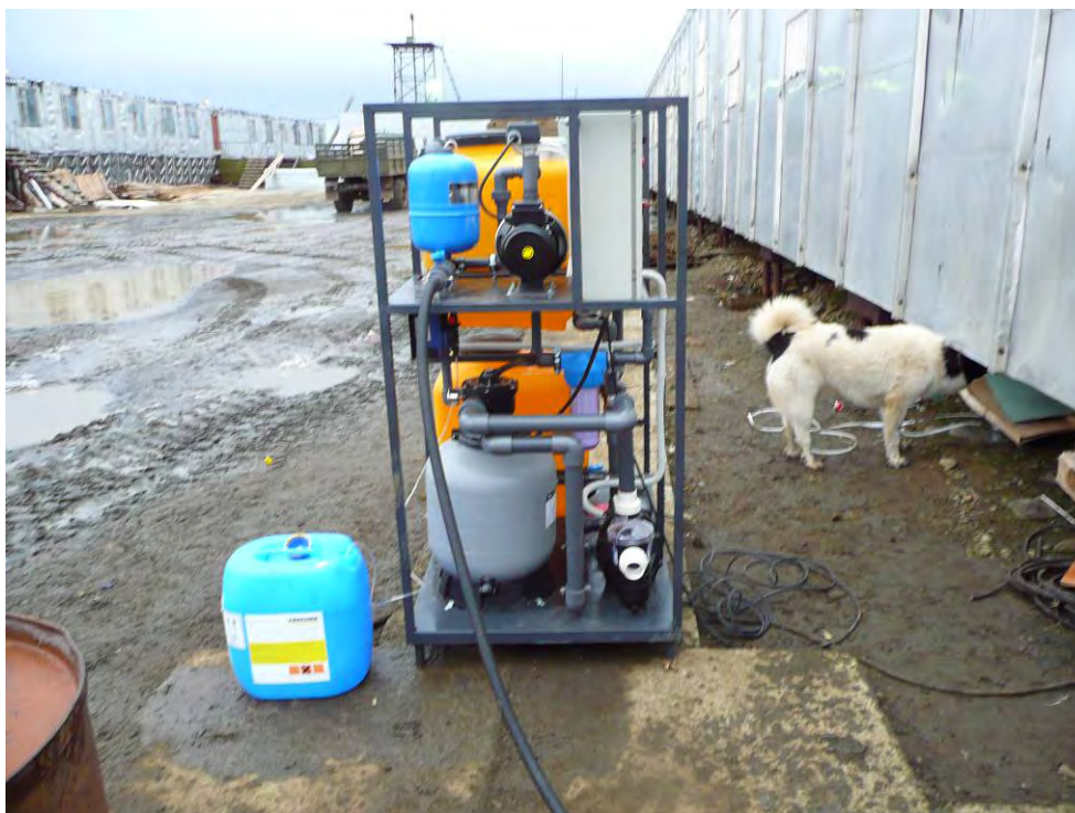
Fig. 6.3.4. "KÄRCHER" washer and water purifying system assembled
