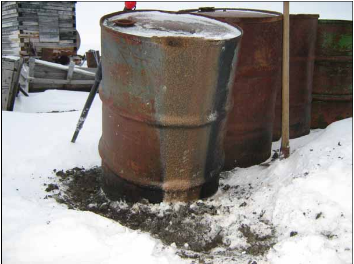
Photo 5.8 Leak of fuel and lubricants near the Diesel plant building
