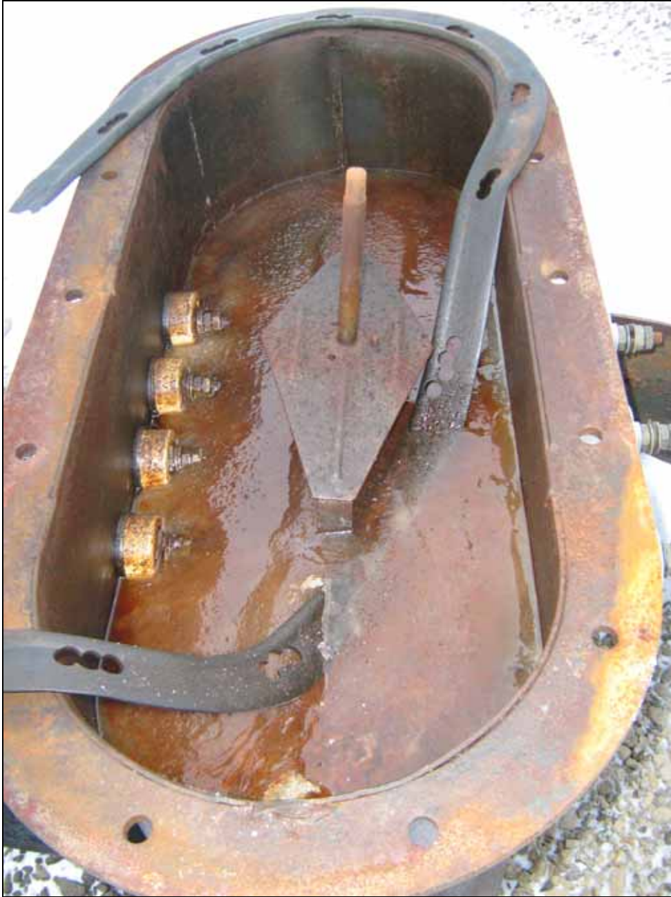
Photo 5.42 Transformer (top view)
