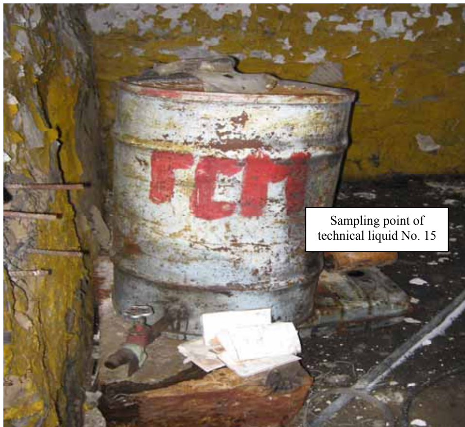
Photo 5.21 Drum in the Diesel station building
