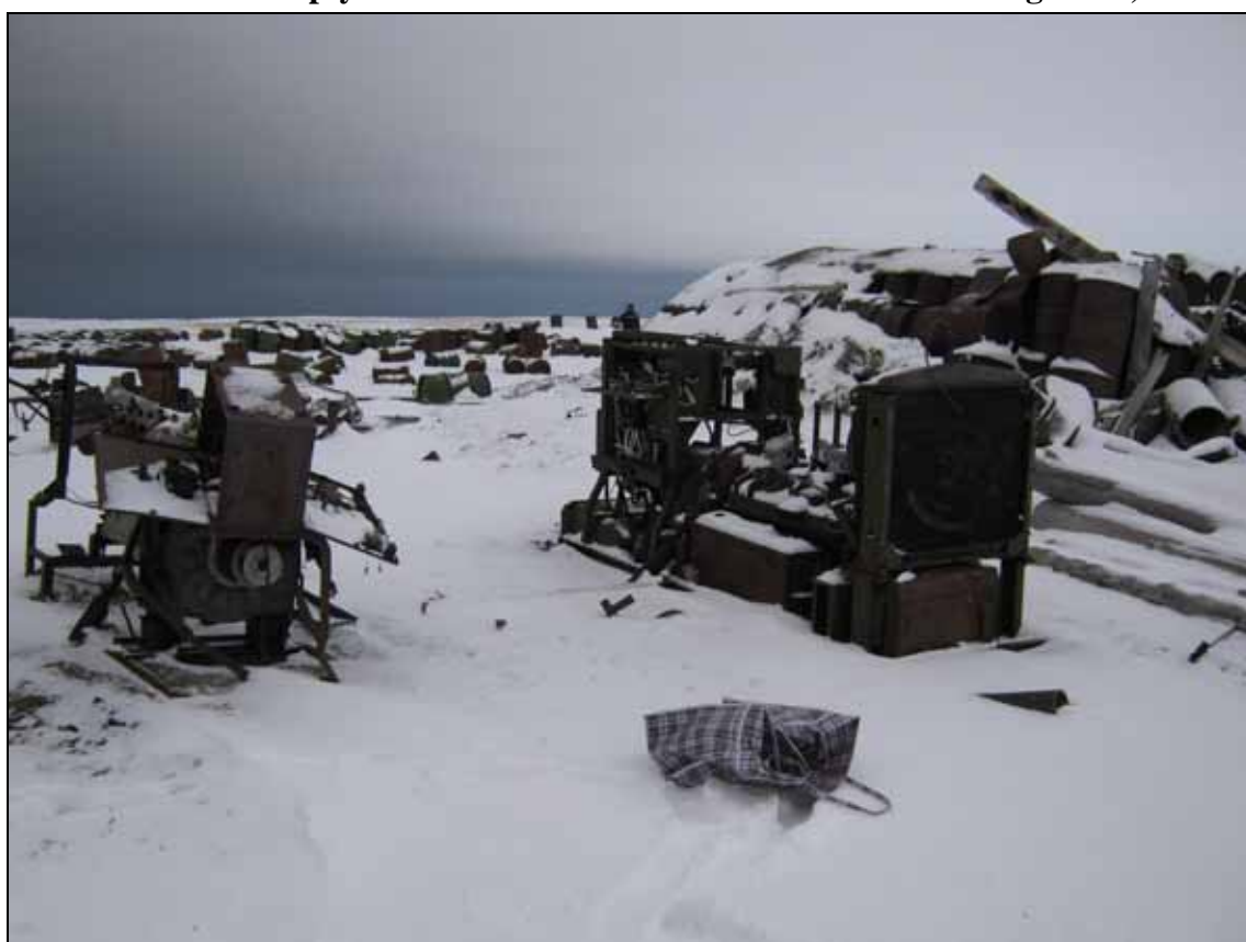
Photo 5.15 Two damaged Diesel generators
