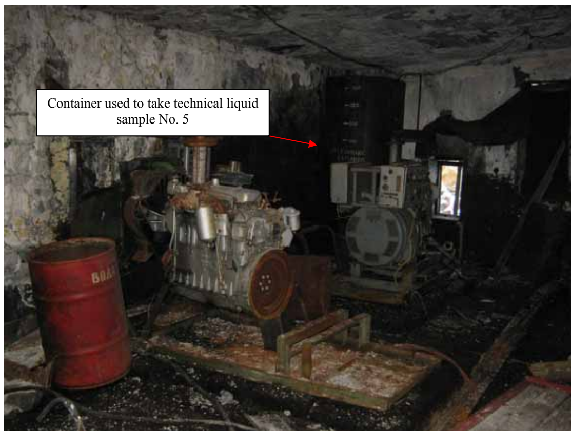
Photo 4.6 Inside the Diesel plant building
