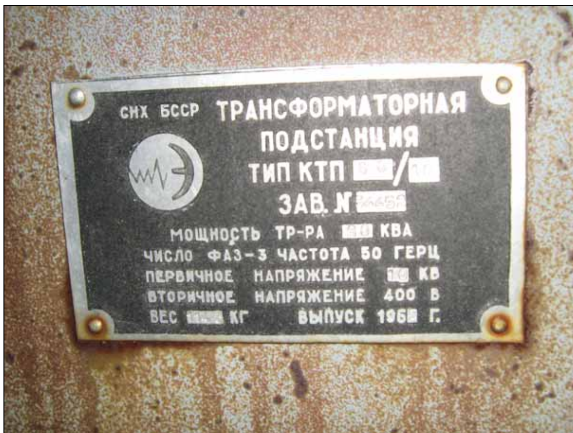
Photo 5.6 Tablet on transformer
