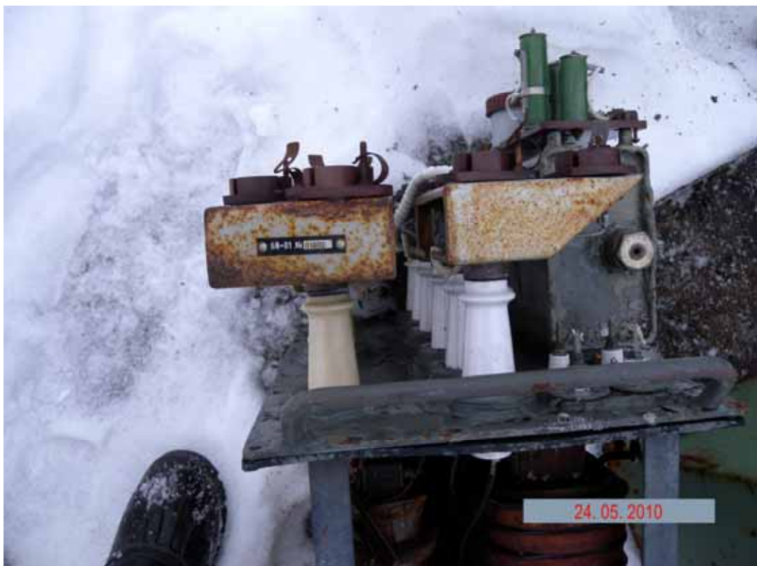
Picture 3.1.13 High-voltage current transformer at the transformer dump (site330) in the surveyed area of the radar station
