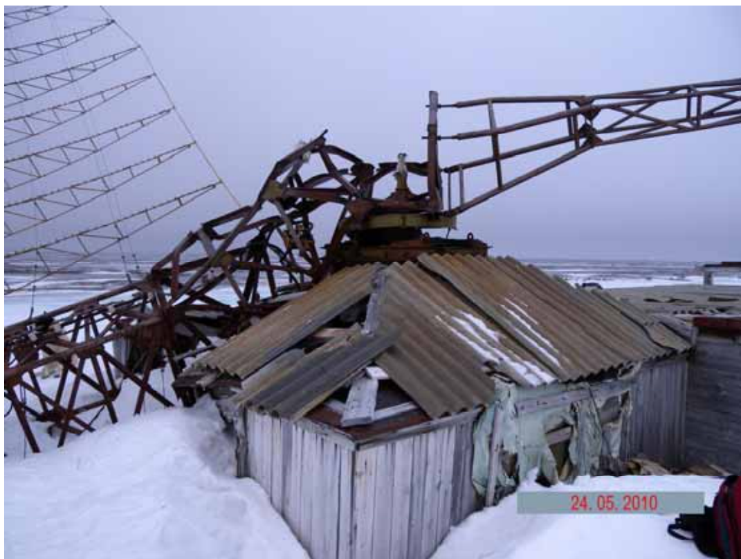
Picture 2.2.33 Antenna and radar station building (items No. 169, 170) in the surveyed area of the radar station
