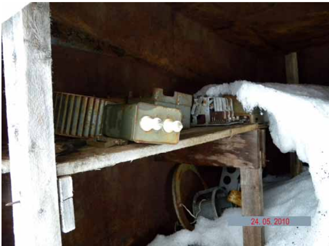
Picture 2.2.30 PCB-containing inside the condenser and transformer storage facility in the surveyed area of the radar station
