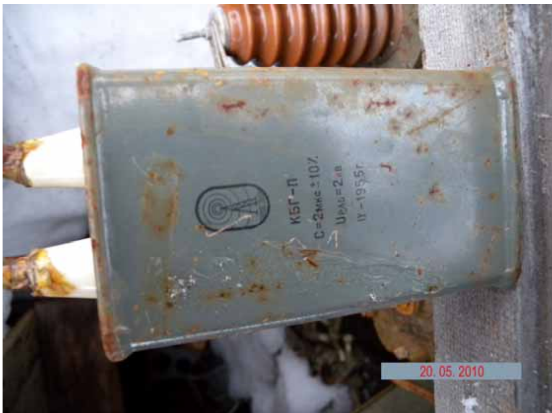
Picture 3.1.3 High-voltage condenser at the condenser and transformer storage facility (site 164) in the surveyed area of the radar station
