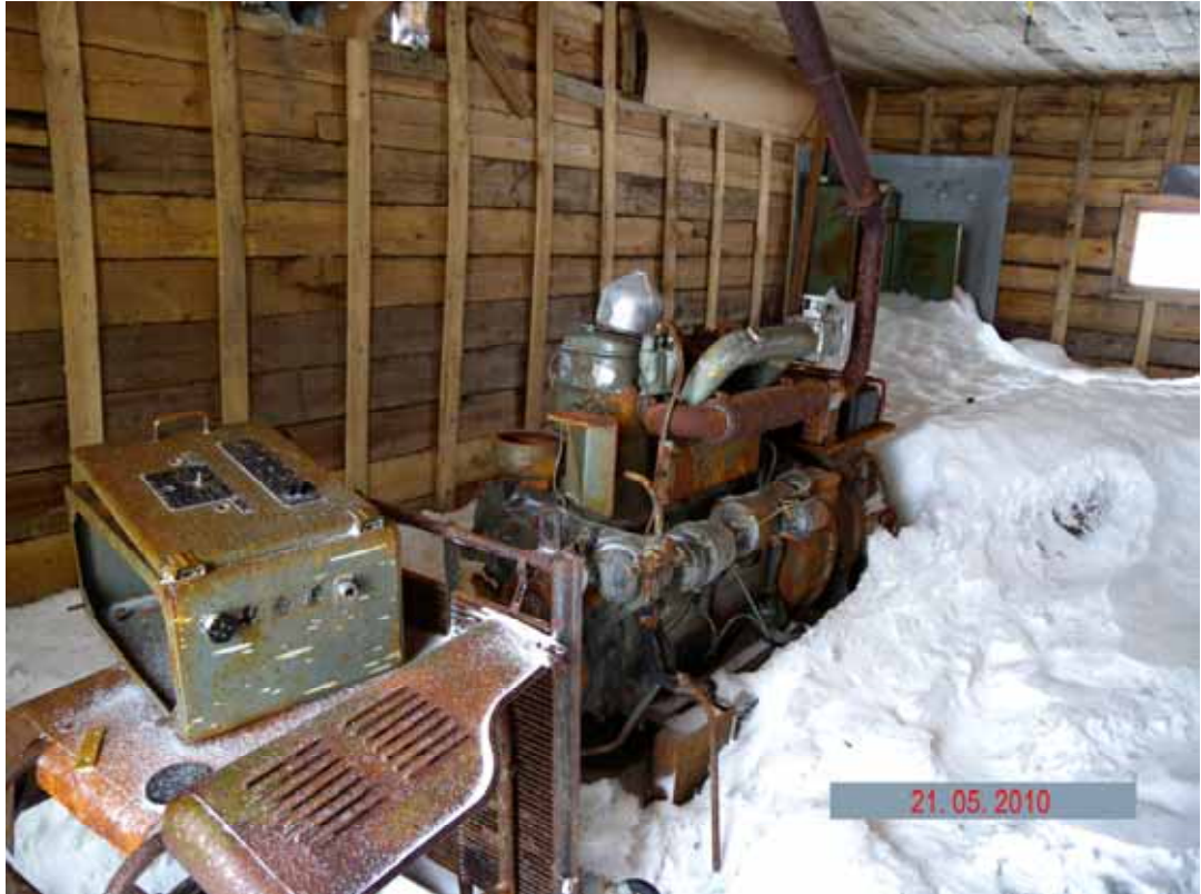
Picture 2.2.17 Diesel generator room (site 280) in the territory of the abandoned polar station
