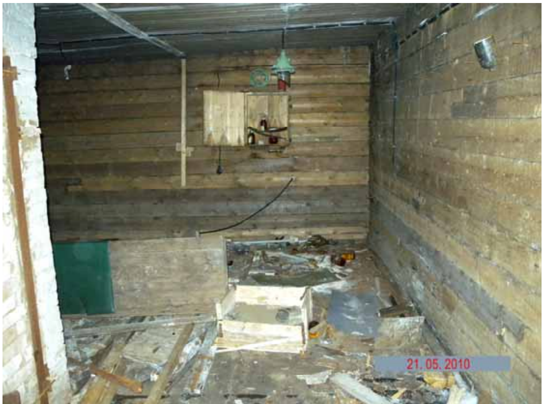
Picture 2.2.18 Room inside the diesel building with chemical agent (site 280) in the territory of the abandoned polar station
