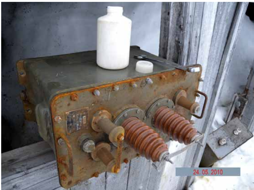
Picture 3.1.5 Radar station high-voltage equipment at the condenser and transformer storage facility (site 164) in the surveyed area of the radar station
