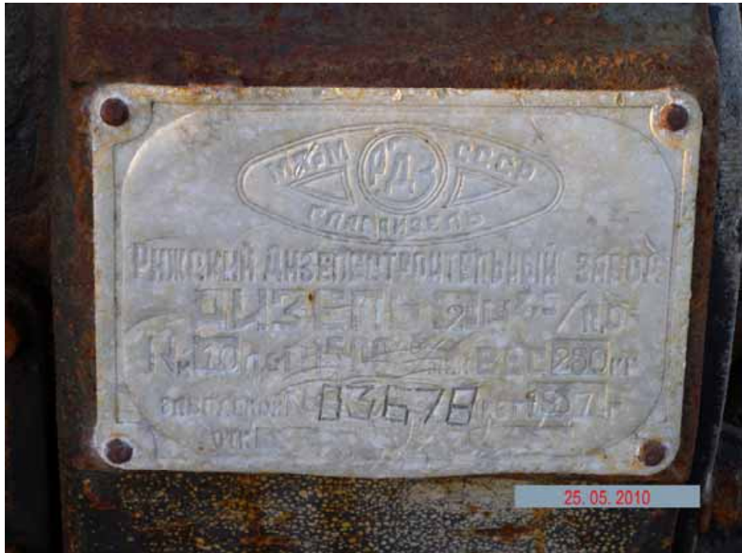
Picture 3.1.14 Diesel power station at the radar station equipment dump in the surveyed area of the radar station
