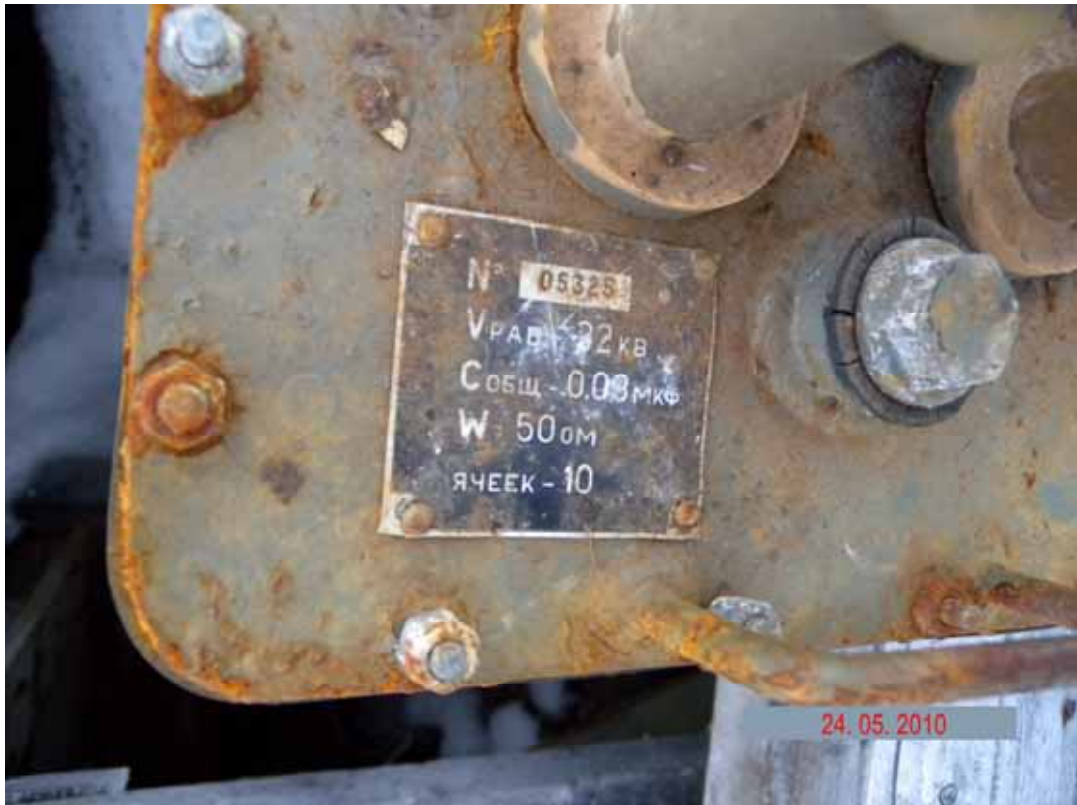
Picture 3.1.6 Radar station high-voltage equipment at the condenser and transformer storage facility (site 164) in the surveyed area of the radar station
