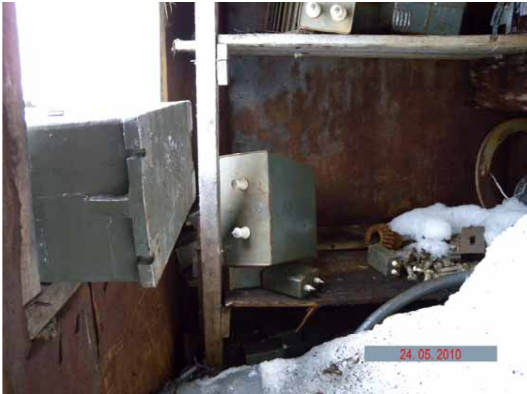
Picture 2.2.31 PCB-containing inside the condenser and transformer storage facility in the surveyed area of the radar station
