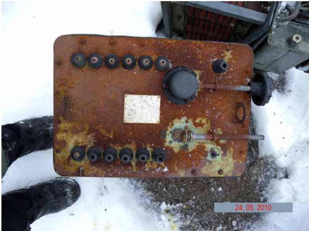
Picture 3.1.12 High-voltage current transformer at the transformer dump (site330) in the surveyed area of the radar station
