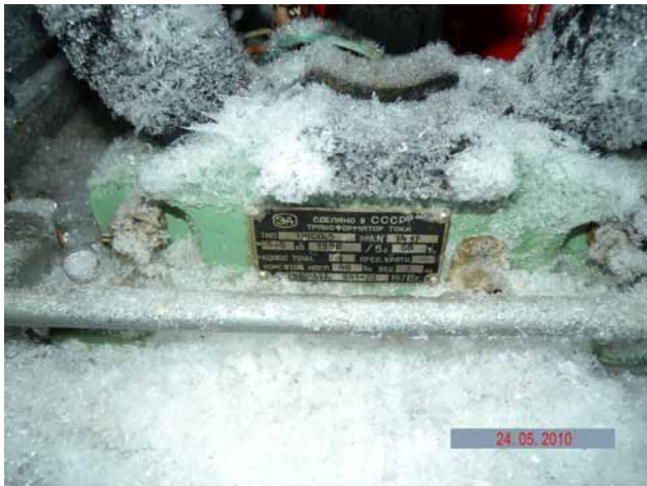
Picture 3.1.11 High-voltage current transformer at the transformer dump (site330) in the surveyed area of the radar station
