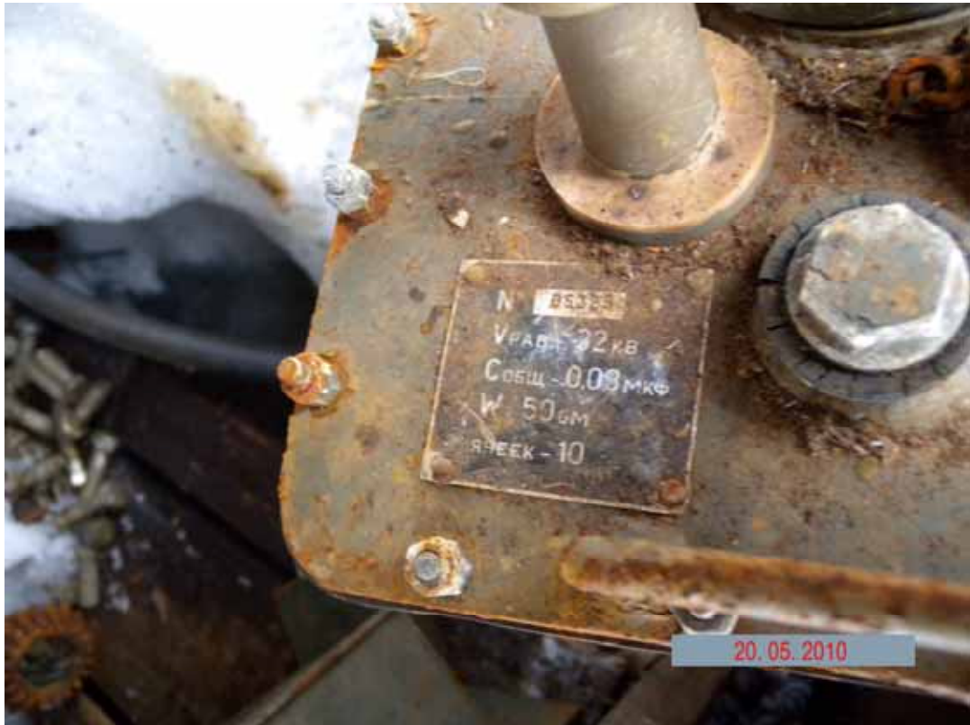
Picture 3.1.2 Radar station high-voltage equipment at the condenser and transformer storage facility (site 164) in the surveyed area of the radar station
