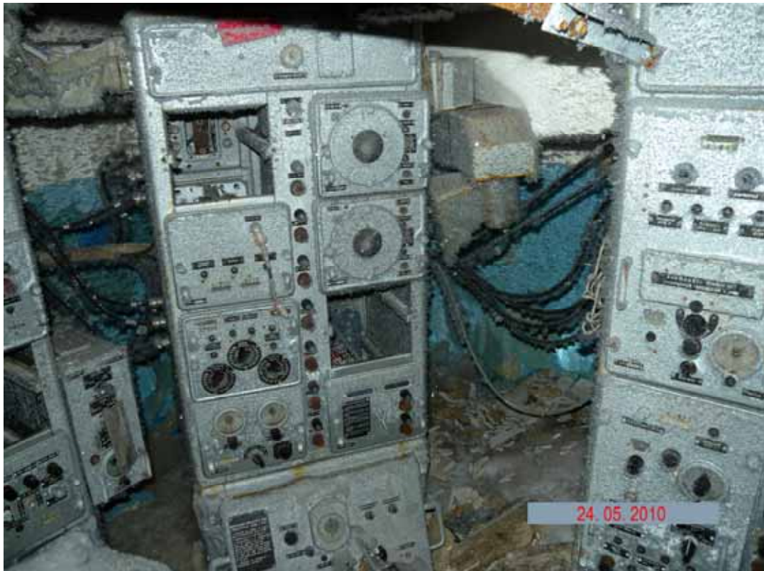
Picture 3.1.8 Radar station equipment in the radar station (site 169) in the surveyed area of the radar station
