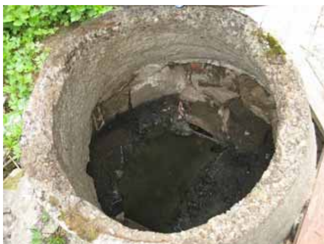
Photo 9. Sewage well at the top point of the overpass
