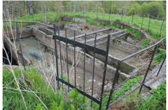
Photo 2. Two-layer settlement tank No.2, filled with sediment
