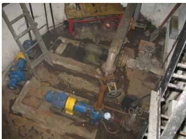
Photo 7. Engine room of the sewage pumping station
