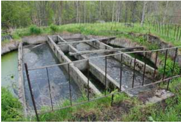
Photo 1. Two-layer settlement tank No.1, in operation
