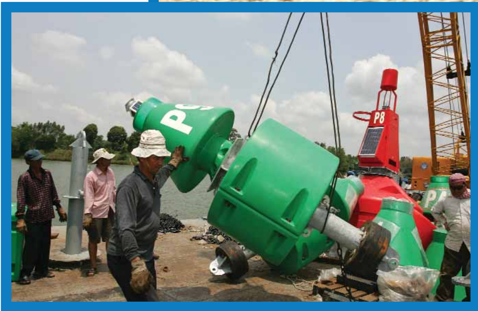
The Navigation Programme has successfully installed a series of buoys, beacons and shoremarks between Phnom Penh Port and the Viet Nam border to assist effective and safe waterborne transport.
