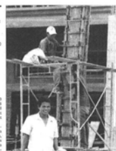
A building site in Phnom Penh. The government is planning to significantly increase spending on the construction of public infrastructure over the next three years. PHNOM PENH
