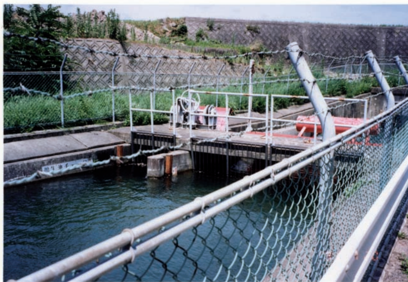
Figure 5.7 Automatic gate (control of water level upstream) accompanied by a manual gate
