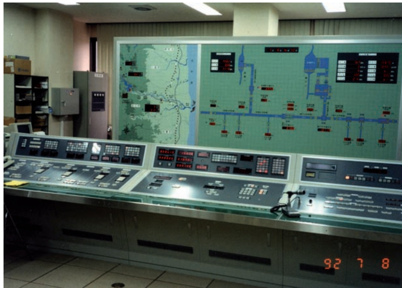
Figure 5.6 A centre for remote monitoring and control
