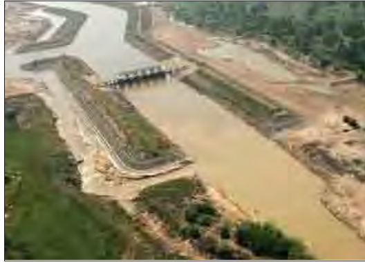
Plate 17. One of the two dams recently built on the middle Songkhram River to divert water for irrigation.
