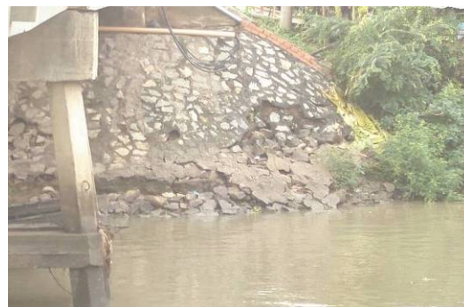
Figure 7 Damage to a bridge abutment.
