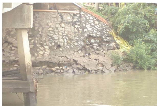
Figure 5.22 Damaged bridge abutment PR855.
