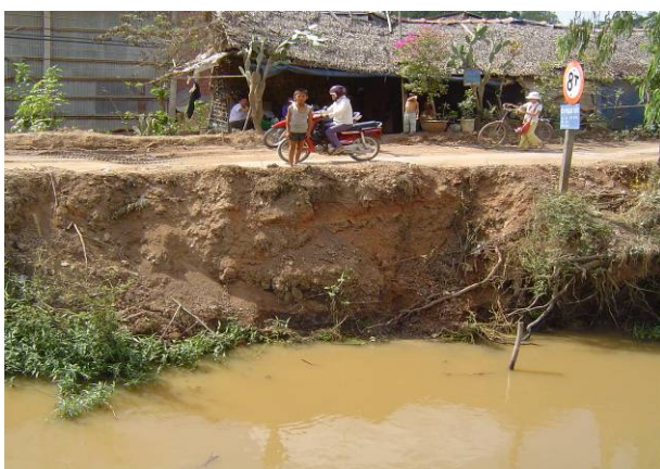
Figure 5.21 Sliding of PR855 after the 2007 flood.
