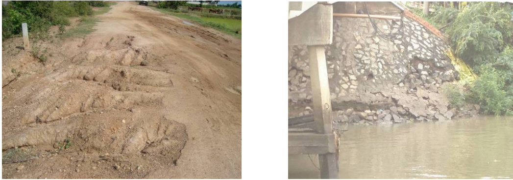
Figure 2.4 Examples of damage due to floods; damage to an unpaved road (left) and damage to a bridge abutment (right).
