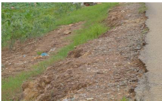
Figure 5.15 Road slope damaged due to flood wave.
