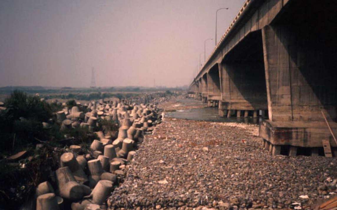
Kaoping River Bridge, Taiwan. Failed from mining-induced incision
