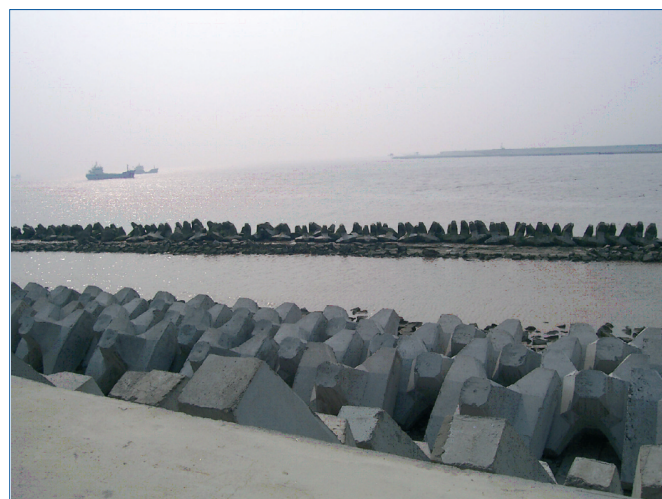
Dikes along the Yangtze coast designed to prevent coastal erosion from reduced sediment input, typhoons and high tides (Photo: M.T. Li)
