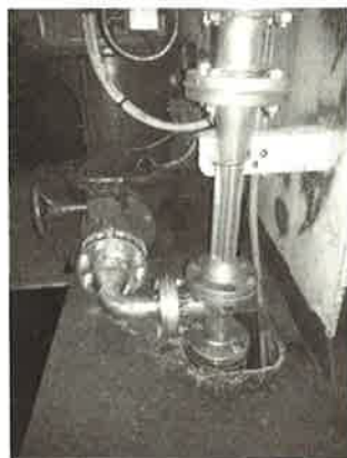
Figure 2. Photograph of installed eductor
