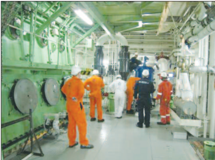
Figure 2. UBWTS installed on “Berge Danuta” (Source-Wilhelmsen Group)
