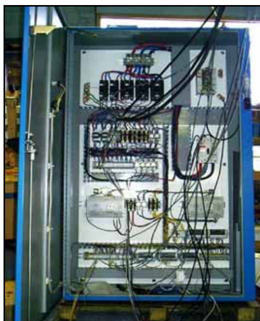
Figure 12. Electrolysis module power cabinet - one of four power and control cabinets.
