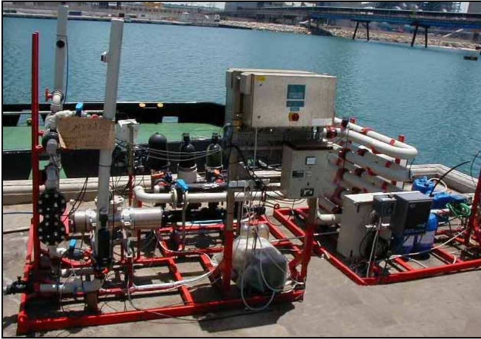
Figure 2. Model I BWT Pilot Unit-General view.
