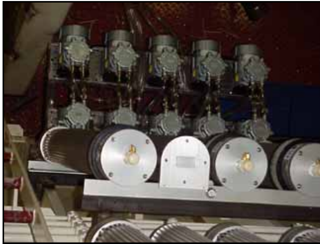
Figure 7. Racks of ionization generators (30) on Carnival Elation pilot project.
