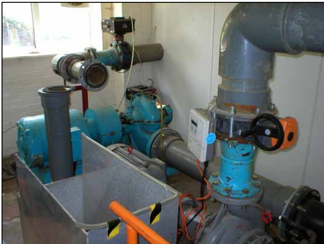
Figure 2. Pumping Facility with total capacity of 400 m 3 /hour.
