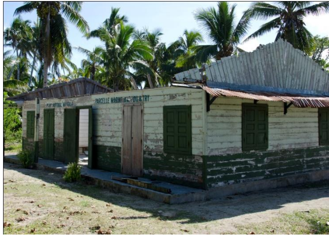
Figure 16: The Masoala National Parks office in Ambodiletra with the damaged roof
