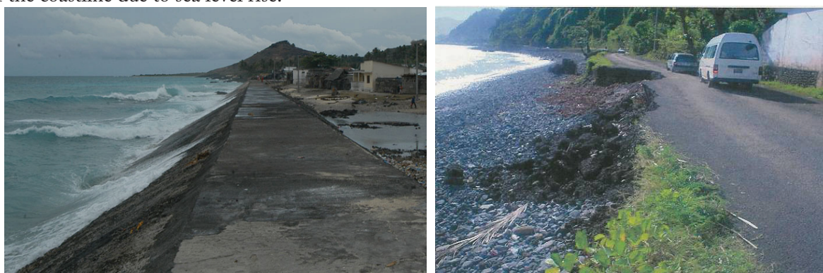
Figures 4: (a) Coastal defence sea wall built to protect the coast against erosion and (b) erosion of the coastline threatening a road.
