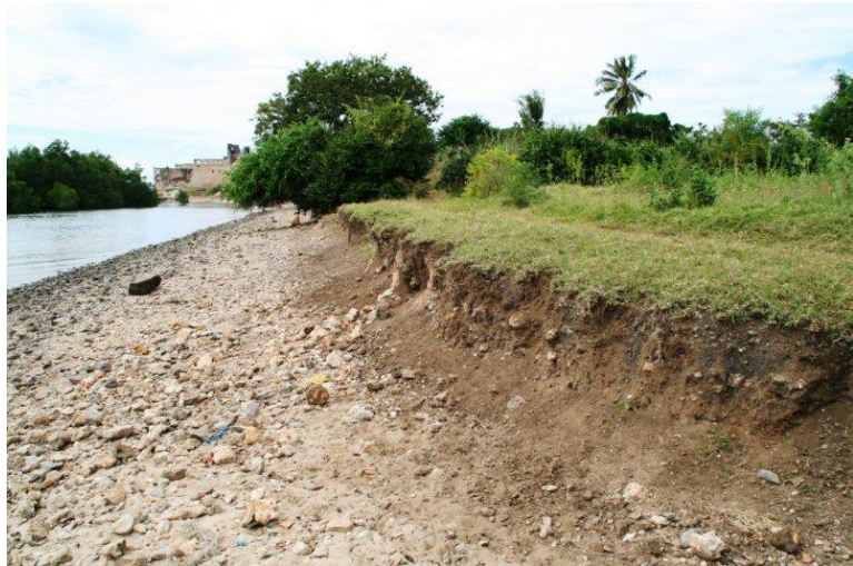
Figure 4: Coastal erosion along the shoreline poses a serious threat to the ruins of Kilwa Kisiwani.
