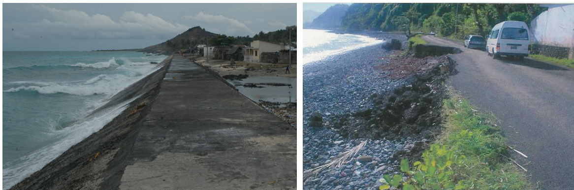
Figures 4: (a) Coastal defence sea wall built to protect the coast against erosion and (b) erosion of the coastline threatening a road.
