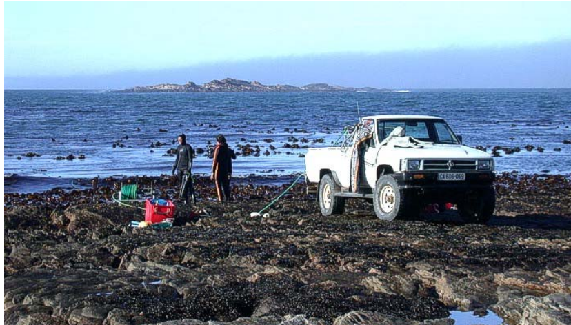
Plate 6. Low pressure compressor located on a vehicle on the shore, and airline feeding down to a pneumatic drill used to install collectors and collector base-plates.
