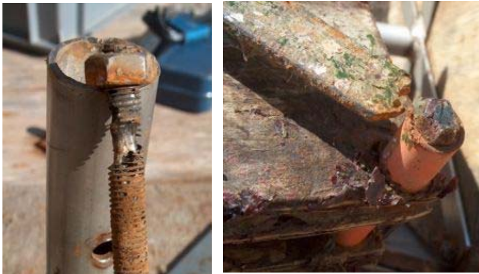
Plate 12. Corrosion of galvanised steel collector bolts and cross-pieces.
